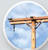
Utility cross arms
